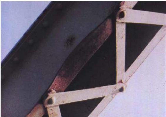
Fonte: BRIDGE INSPECTION MANUAL – NY'S DOT
