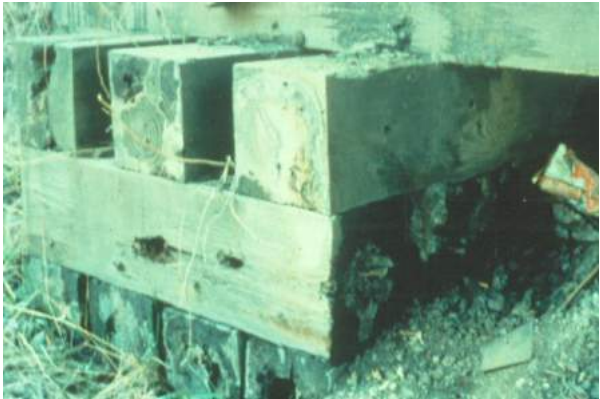
Fonte: BRIDGE INSPECTION MANUAL – NY'S DOT
