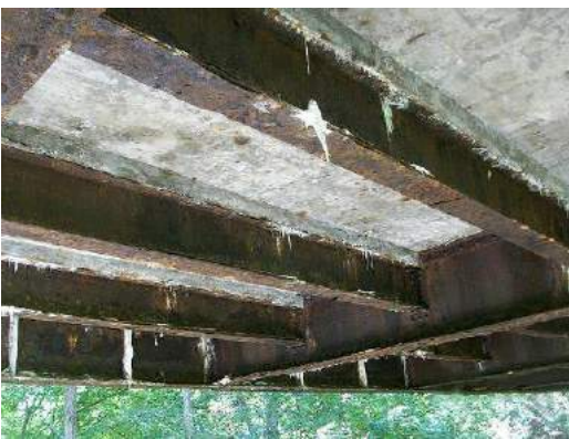
Fonte: BRIDGE INSPECTION MANUAL – NY'S DOT
