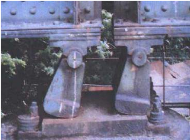
Fonte: BRIDGE INSPECTION MANUAL – NY’S DOT
