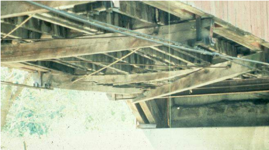
Fonte: BRIDGE INSPECTION MANUAL – NY’S DOT
